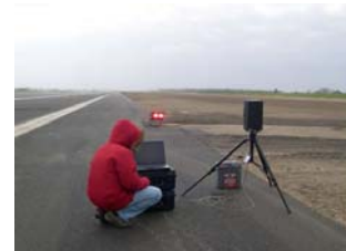
ACS field engineer using state-of-the-art PAPI Calibration equipment
